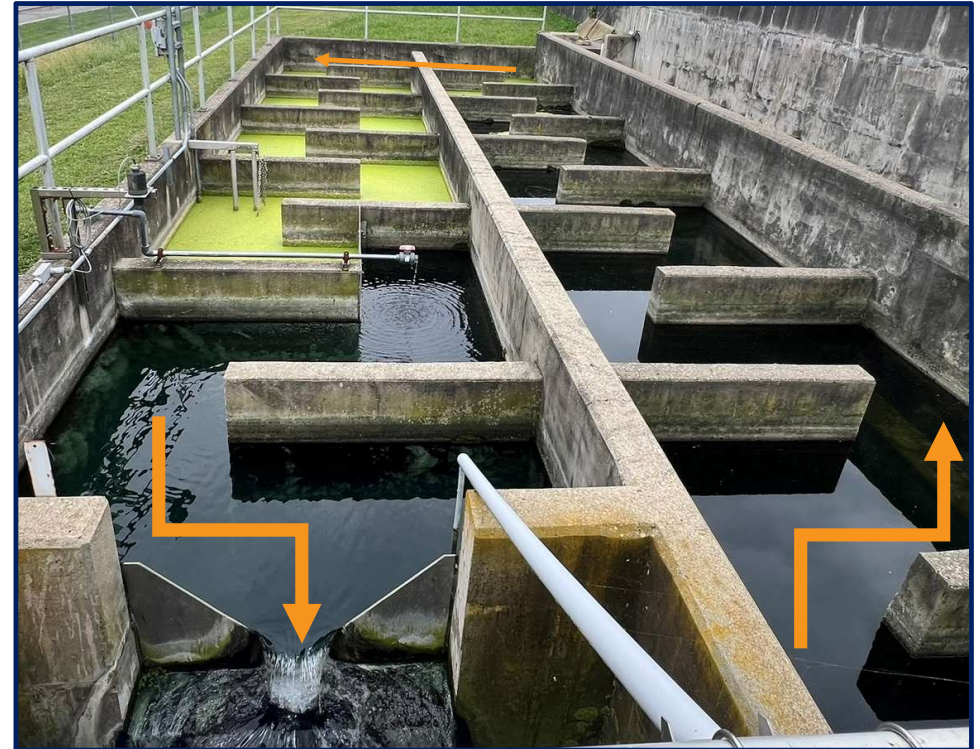
Outgoing flows are disinfected and measured before release
