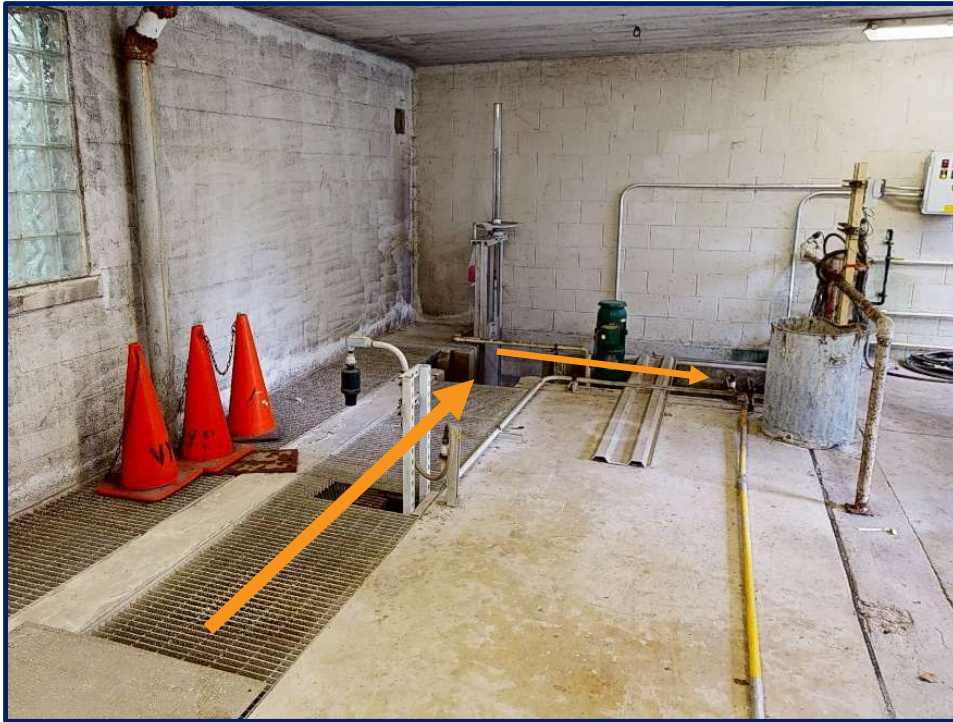
Main collection site where flows are measured and recorded before passing through a grinder pump to break down solids
