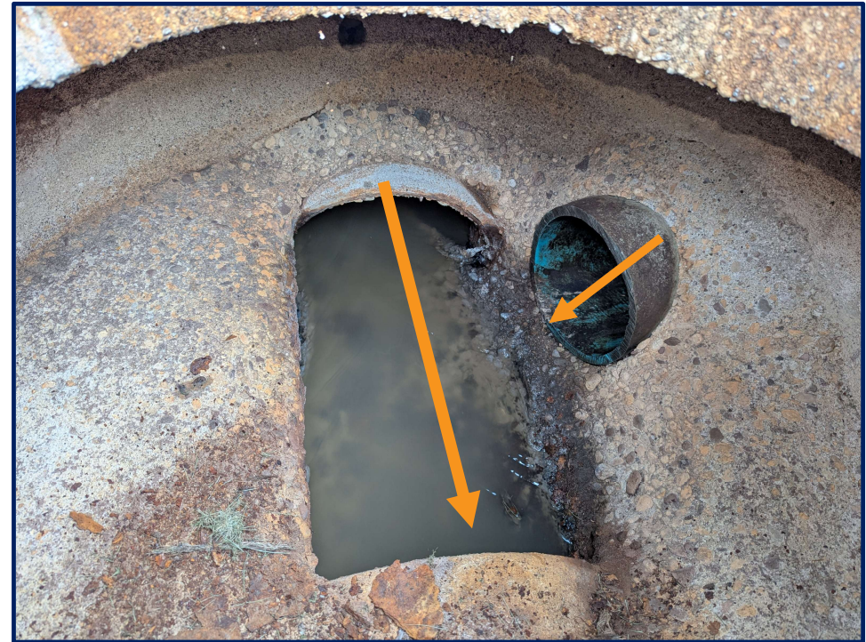
Pressurized flow from the force main discharges into the main gravity sewer carrying wastewater to the treatment plant
