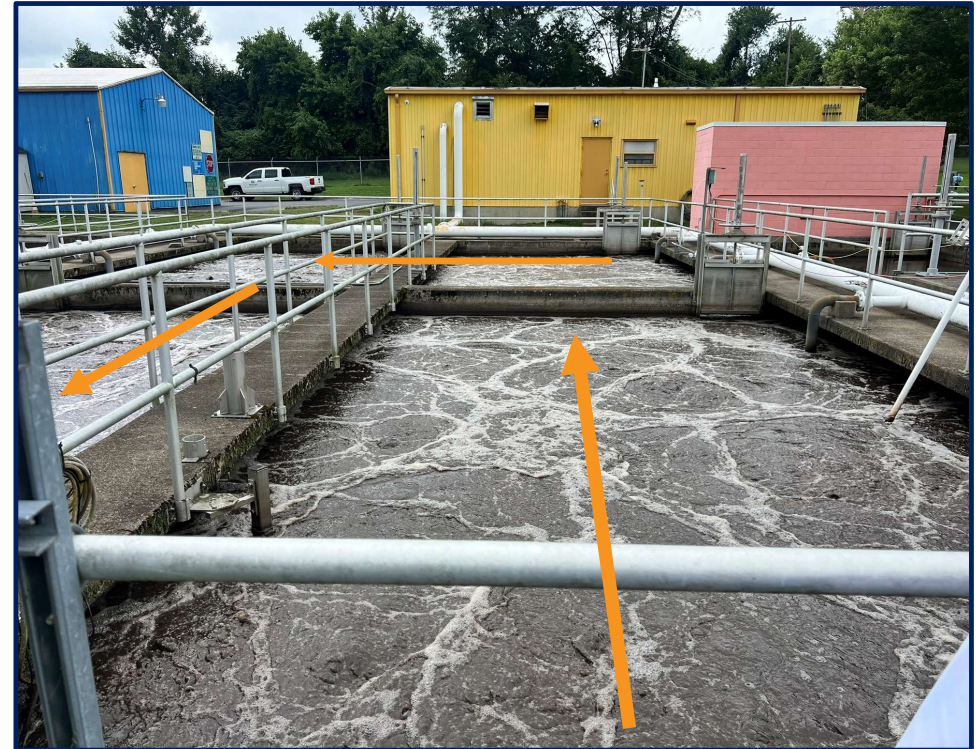
Air supports bacteria to break down waste and remove nutrients
