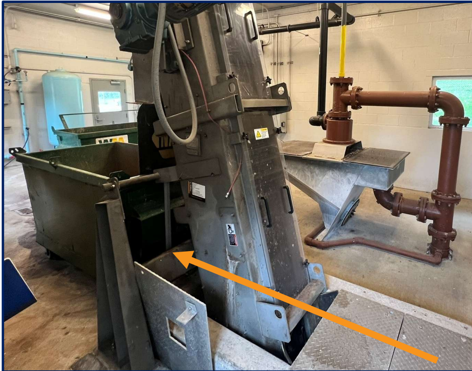
Screens remove large debris before further treatment
